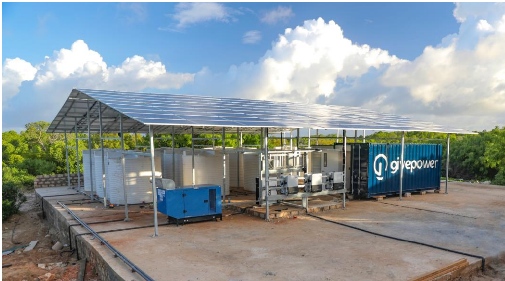
Figure 5: Solar powered desalination plant
