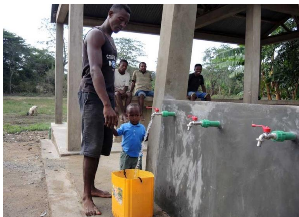
Figure A-2. Example of clean water system constructed under this PoA
